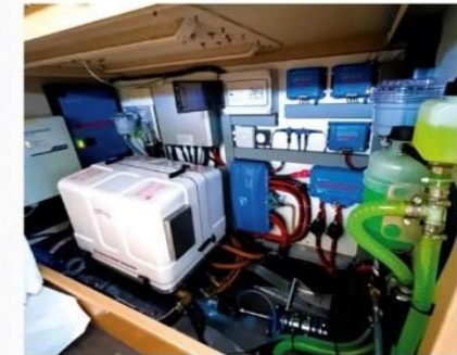
A large technical area includes plenty of space for genset and electronics
